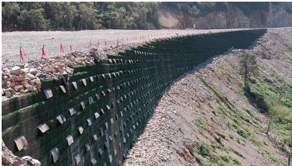
Figure 19. Wall reinforced with geosynthetics.
