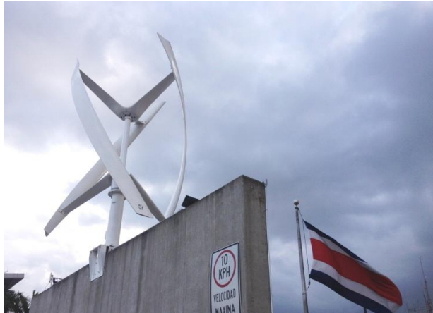
Figure 29: Eolic Generator provides electricity to the parking Source: Picture taken during onsite visit, April 2013
