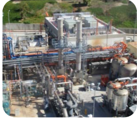
Hyperion Wastewater Reclamation Plant's Digester Gas Utilization Project Los Angeles, CA
