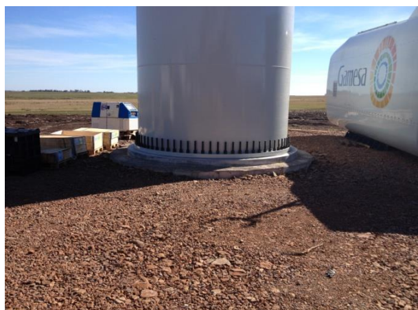
Figure 30: Reuse of excavated material. Source: Picture taken during the onsite visit May 2013
