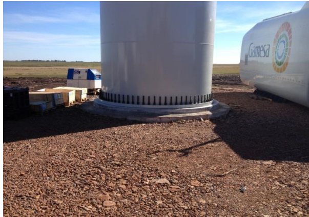
Figure 46: Reuse of the excavated material to fill the top of the foundation Source: Picture taken during the onsite visit May 2013
