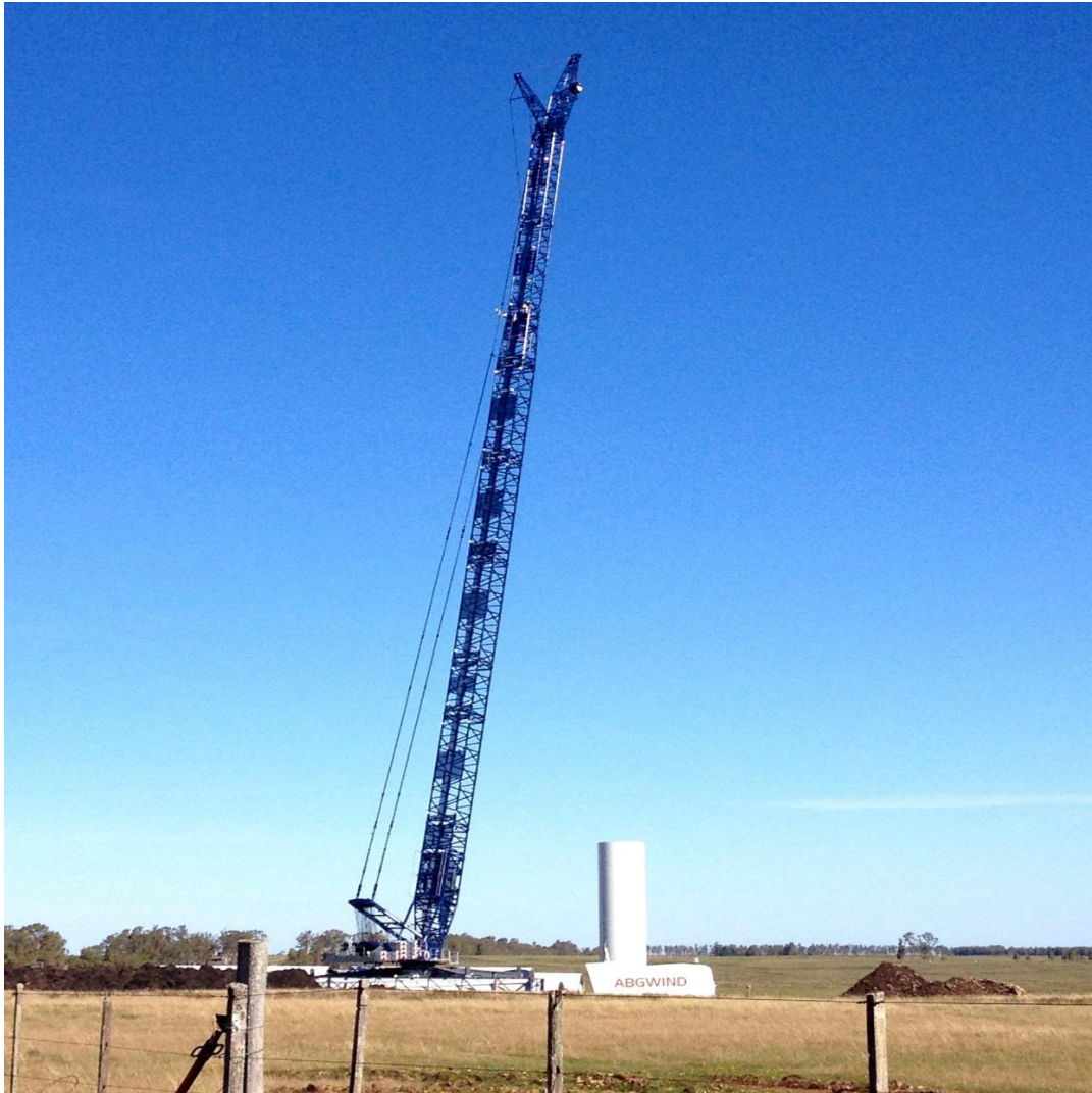
Figure 1: Assembly process of one of the turbines/ Source: Picture taken during onsite visit, May 2013
