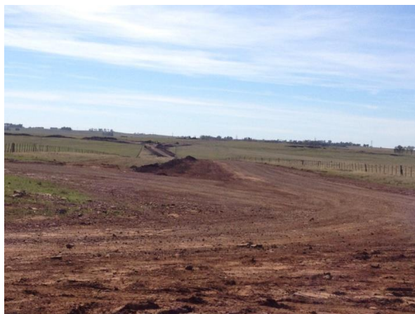
Figure 27: Reuse of excavated material. Source: Picture taken during the onsite visit May 2013
