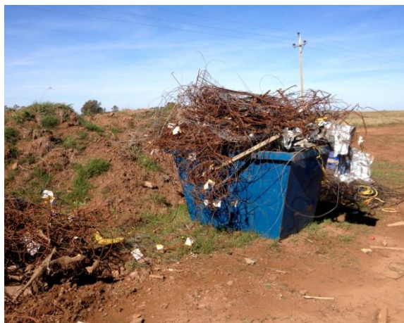
Figure 31: Recycling of the scrap steel from the construction site Source: Picture taken during the onsite visit May 2013
