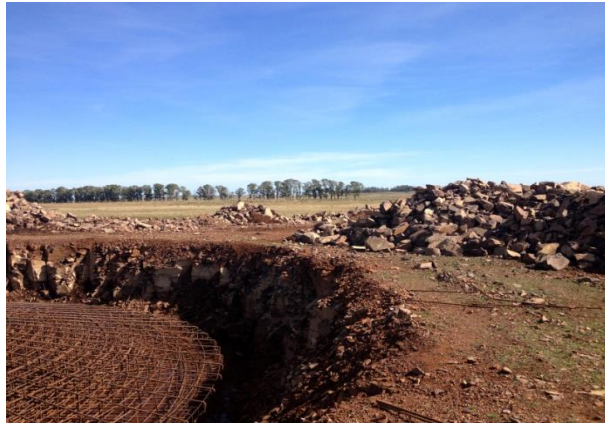
Figure 45: Material storage at the edge of the foundation Source: Picture taken during the onsite visit May 2013
