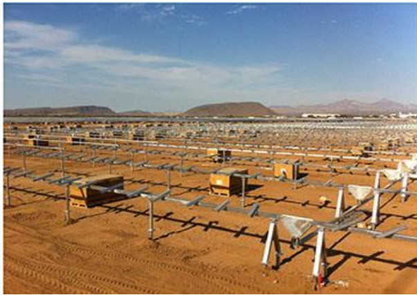
Figure 42: Placement of Module Structure Source: Martifer Solar. PV Aura Solar I 20MW Informe Quincenal, Semana 32-33. August 2013, p. 39.
