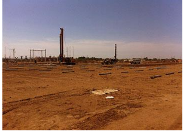
Figure 41: Screw Foundations Set Up Source: Martifer Solar. PV Aura Solar I 20MW Informe Quincenal, Semana 32-33. August 2013, p. 35.
