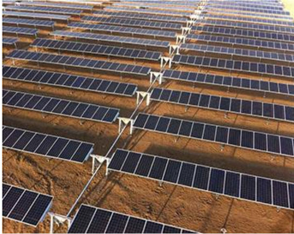
Figure 46: Photovoltaic Module Installation Source: Martifer Solar. PV Aura Solar I 20MW Informe Quincenal, Semana 32-33. August 2013, p. 42.
