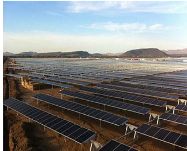
Figure 47: Photovoltaic Module Installation Source: Martifer Solar. PV Aura Solar I 20MW Informe Quincenal, Semana 32-33. August 2013, p. 42.
