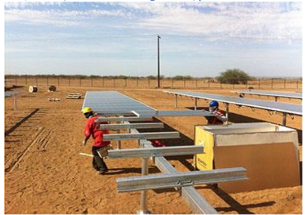
Figure 43: Set Up of Modules on Structure Source: Martifer Solar. PV Aura Solar I 20MW Informe Quincenal, Semana 32-33. August 2013, p. 41.
