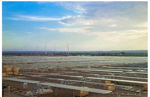
Figure 45: Photovoltaic Units' Set Up with High Tension Line Source: Aura Solar, Línea de Tiempo, p. 7.
