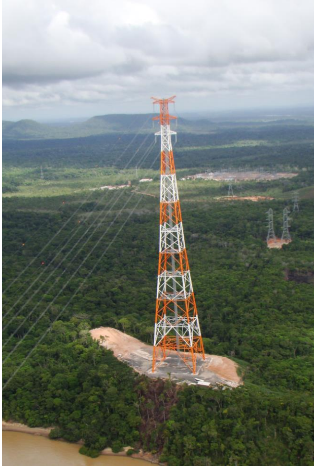
Figure 32: High Tension Towers at the Amazon River / Source: Isolux Corsán
