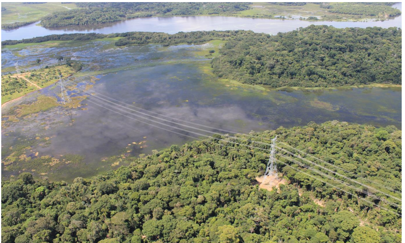
Figure 40: General view of the high tension line / Source: Isolux Corsán
