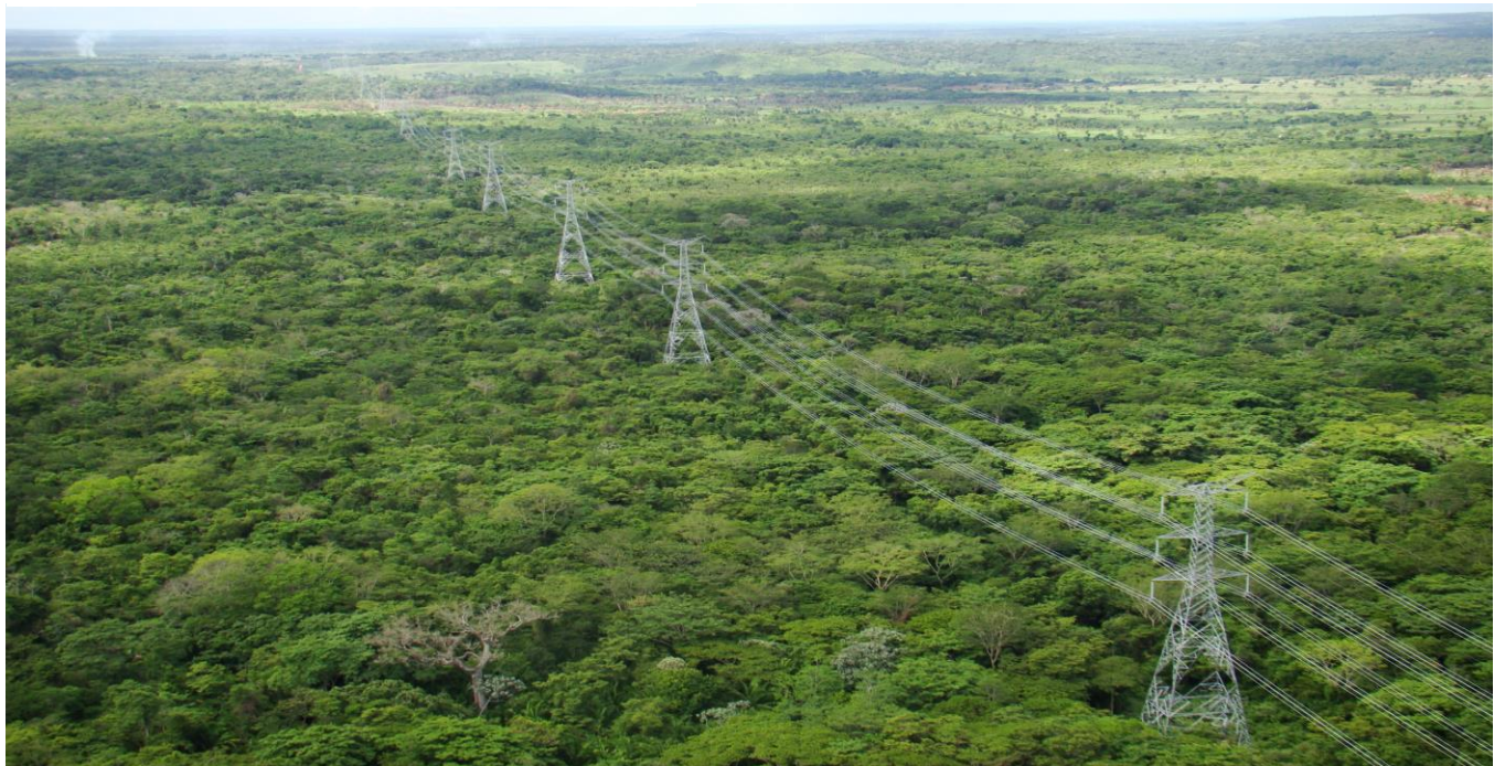
Figure 34: General view of the transmission line through the jungle /. Source: Isolux Corsán
