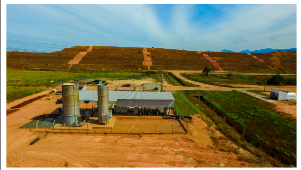
Figure 28: Biogas flare at CTR Rio. Sources: Image sent from CTR Rio project team
