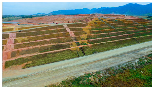
Figure 27: Landfill cells at CTR Rio. Sources: Image sent from CTR Rio project team
