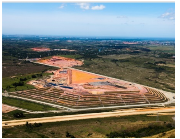
Figure 32: CTR Rio in December 2013. Sources: Image sent from CTR Rio project team
