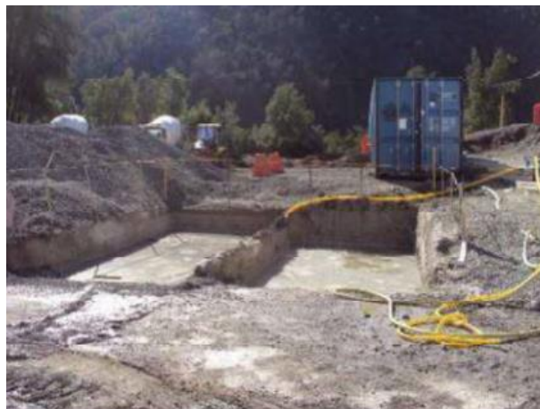
Figure 29: construction of concrete plant with a recirculating water system. Picture provided by Besalco S.A.
