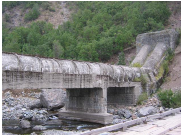
Figure 06: “El Melado Canal”, siphon “El Toro”, 1.2 km route. . Source: Besalco S.A., US department of energy.
