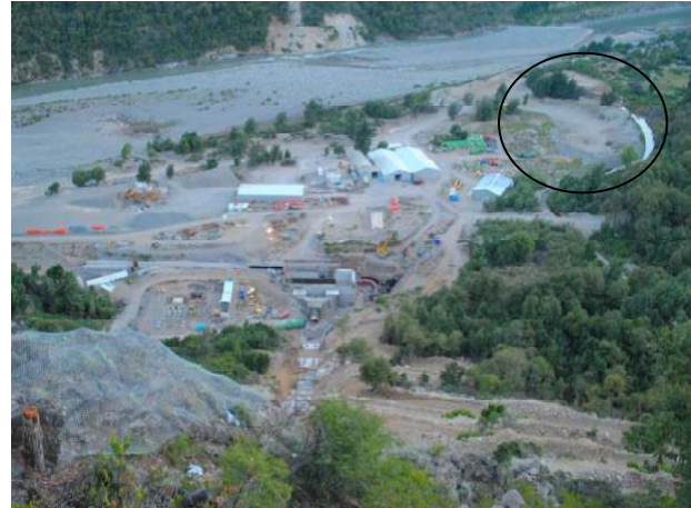
Figure 28: deposits of accumulated material. Picture provided by Besalco S.A.
