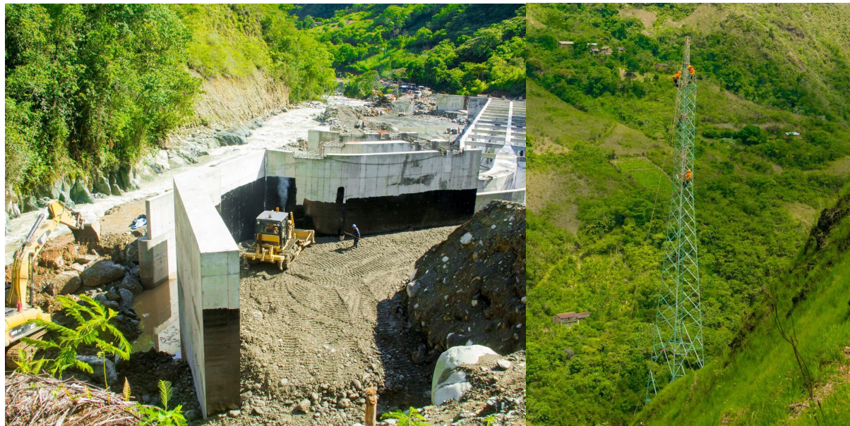
Fig 01: 8 de Agosto hydroelectric plant and 138 kV transmission line Source: Generación Andina S.A.C.
