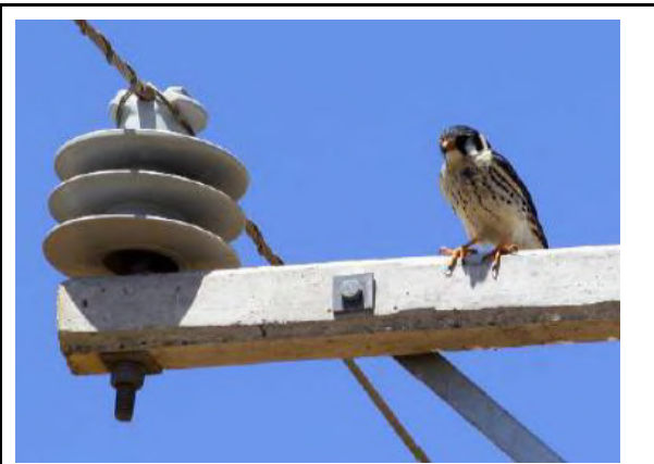
Figure 34: Birds with electrocution risk due to non-isolated structures. Sources: Generación Andina S.A.C.
