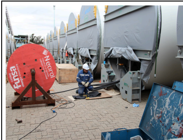
Figure 14: Place where turbines are assembled. Sources: Piñon, A, Polesine S.A., "Componente Nacional de Inversión Parque Eólico Florida." Jul. 29 2013, p. 5.
