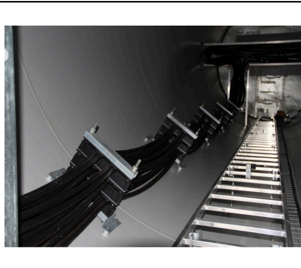
Figure 18: The interior of the towers where all electric wiring and metallic installations have been completed. Sources: Piñon, A, Polesine S.A., "Componente Nacional de Inversión Parque Eólico Florida." Jul. 29 2013, p. 4.
