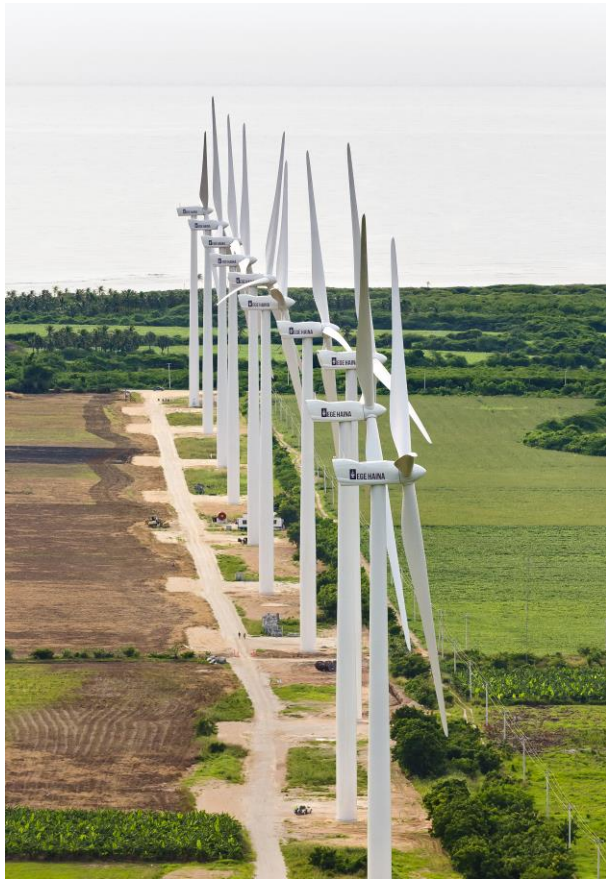
Figure 36: General view of Los Cocos windfarm. / Source: EGE Haina
