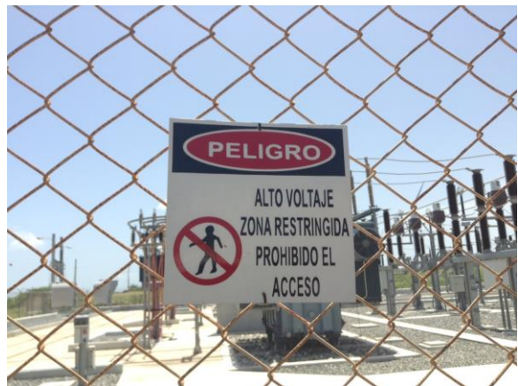
Figure 06 : Sign reading “Danger: High Voltage Restricted Zone Access Prohibited” Source: EGE Haina
