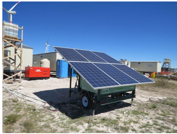
Figure 14: Solar Panels to energize work area Sources: Enel Green Power, "Planta Fotovoltaica Evidencia Fotográfica" [Photographic Evidence], Image Submitted for Envision Evaluation
