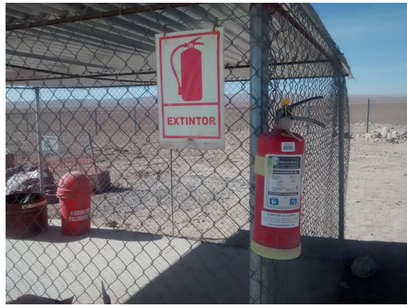
Figure 13: Safety warnings inside the plant Sources: Solarpack
