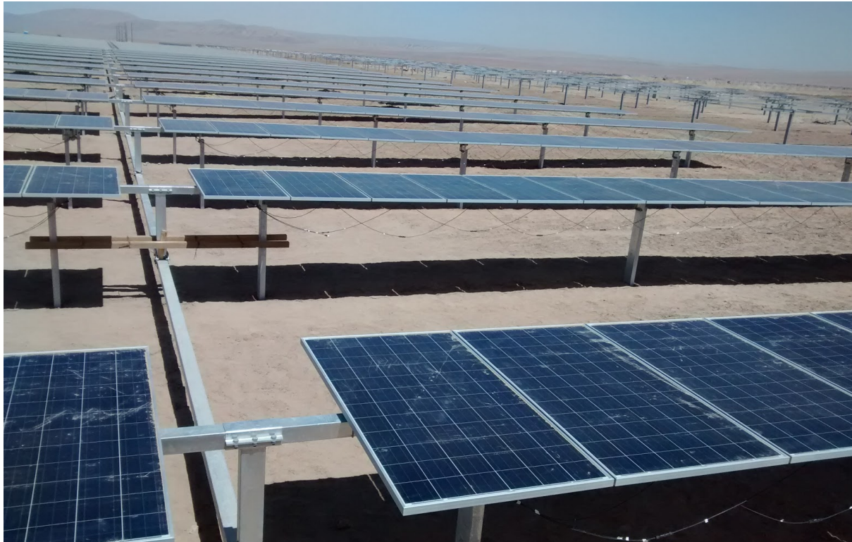
Figure 02: Overview of the plant Sources: Solarpack
