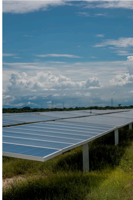
Figure 34: Photovoltaic Modules Relation to the Ground. Sources: Anexo Fotográfico .
