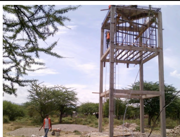
Figure 11: Construction of elevated tank to distribute water to the community by gravity in Colonia Victor Manuel Argeñal I. Sources: Clever Honduras, Informe de Avance Social de Sitio Pacífico I, Choluteca I y II . Semana del 06 al 12 de agosto del 2015 (Choluteca, 2015), 5.
