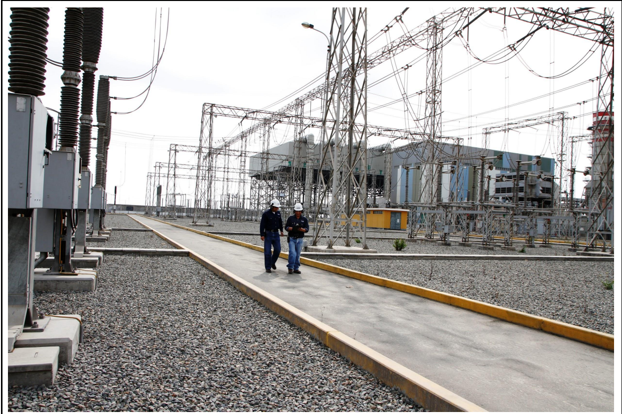
Figure 06: General view of the project. Source: EnerSur.
