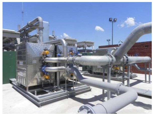
Figure 11: Siloxane Removal Plant
