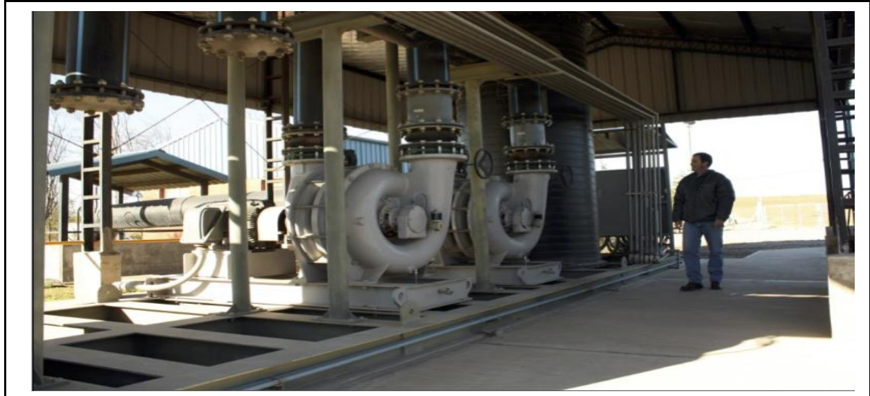
Figure 5: General picture of the project, Biogas Capture Plant
