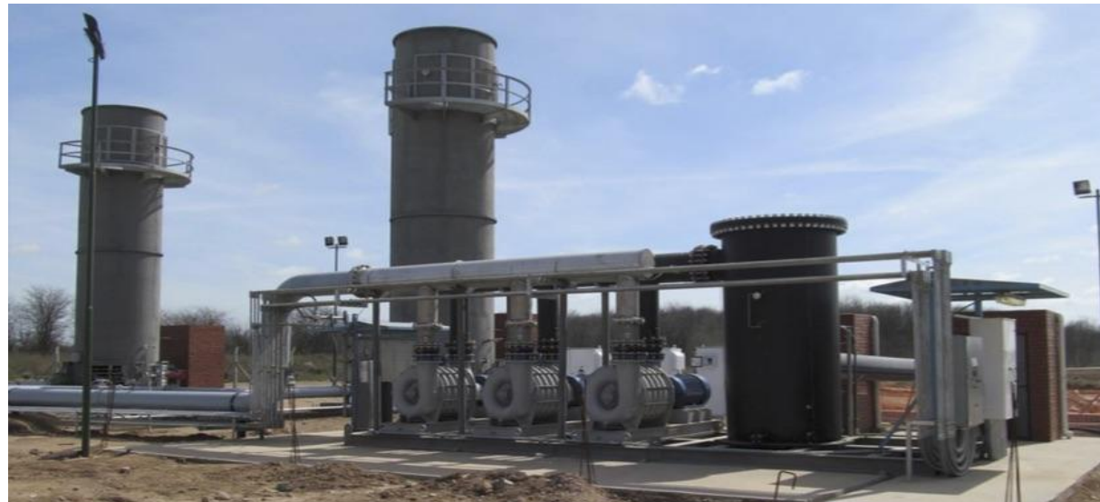
Figure 13: Biogas Capture System
