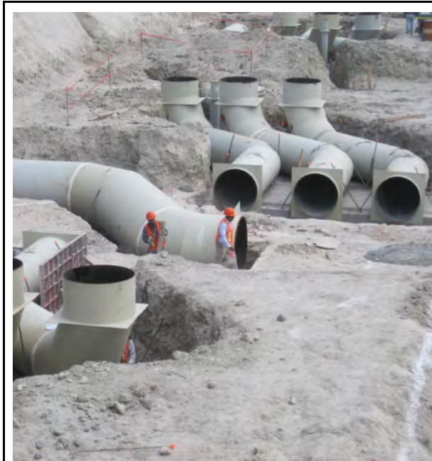
Figure 14: Photo of the construction works. Sources: SEMARNAT. Planta de Tratamiento de Aguas Residuales Atotonilco . Mexico: 2014.
