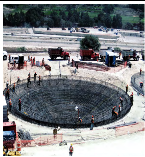
Figure 15: Photo of the construction works. Sources: SEMARNAT. Planta de Tratamiento de Aguas Residuales Atotonilco . Mexico: 2014.
