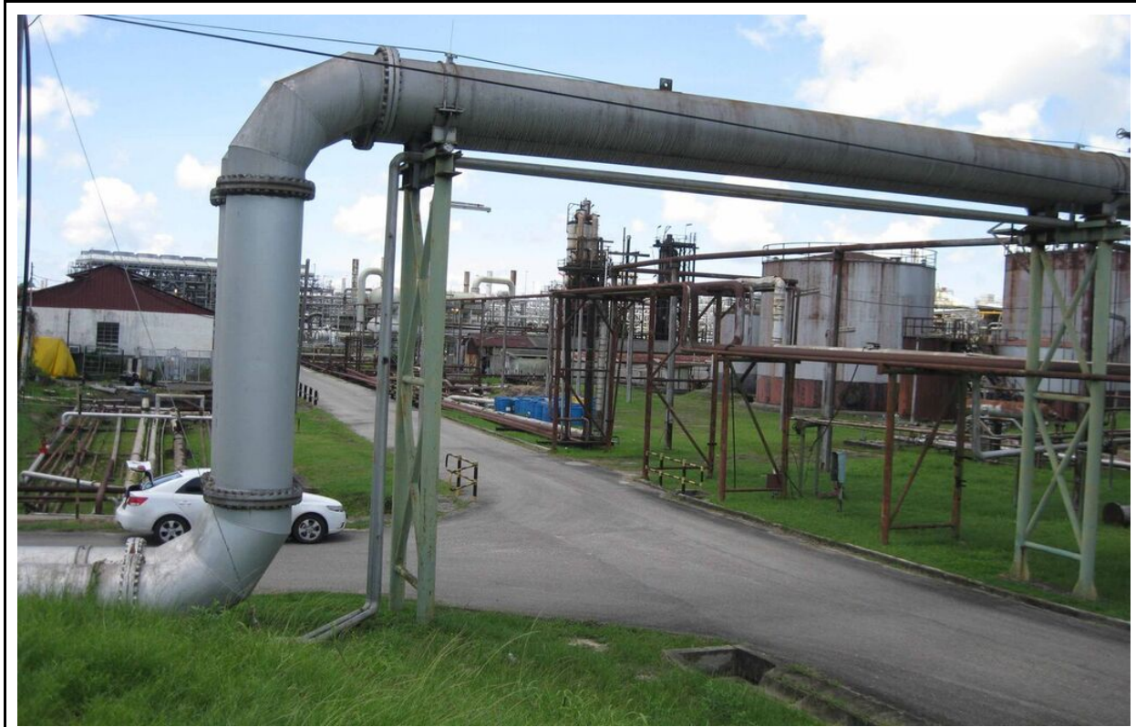
Figure 9: Pipes to the Sea to Aquastore to the Tanks Sources: Images Seven Seas Water Company "Pipes 2010-09-01"
