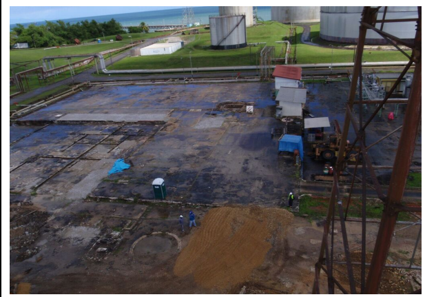
Figure 15: The Site after Clean-up Sources: The Site after clean-up, Dropbox Delivered by Seven Seas Water
