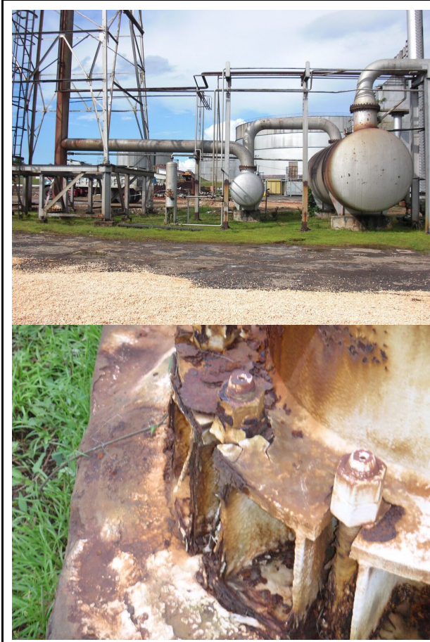
Figure 18 and 19 Structural Photos Sources: Structural Photos by Seven Seas Water and Fire Stack
