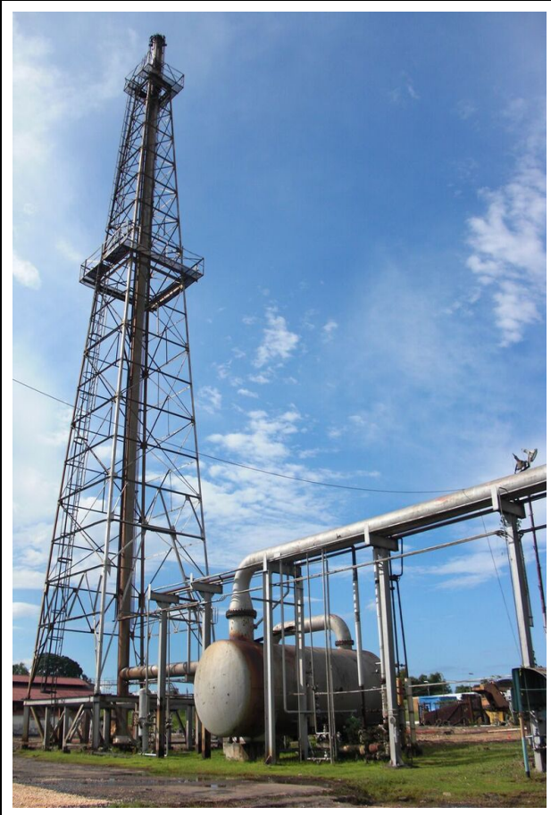
Figure 20: Pipes Sources: Fire Stack by Sven Seas Water
