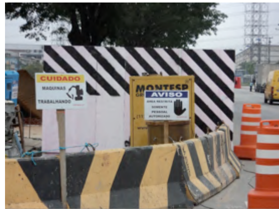
Figure 24: Safety and wayfinding signage in the construction site. Sources: Odebrecht Ambiental, Evidências Fotográficas ( September 5, 2011).
