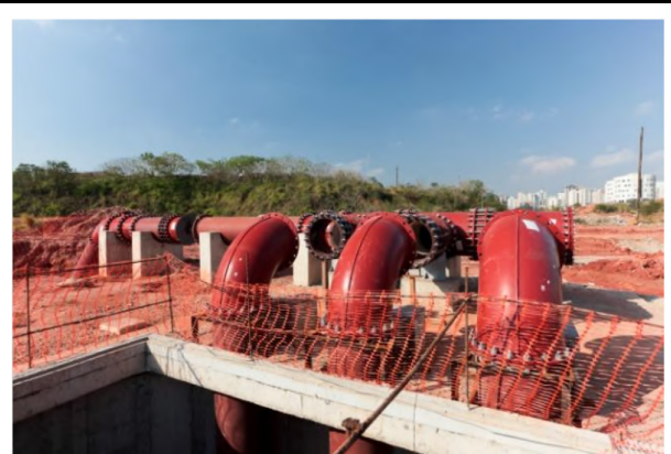
Figure 18: Low charge pump station. Sources: Aquapolo Ambiental, Apresentação geral.
