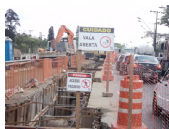
Figure 23: Safety and wayfinding signage in the construction site. Sources: Odebrecht Ambiental, Evidências Fotográficas ( September 5, 2011).
