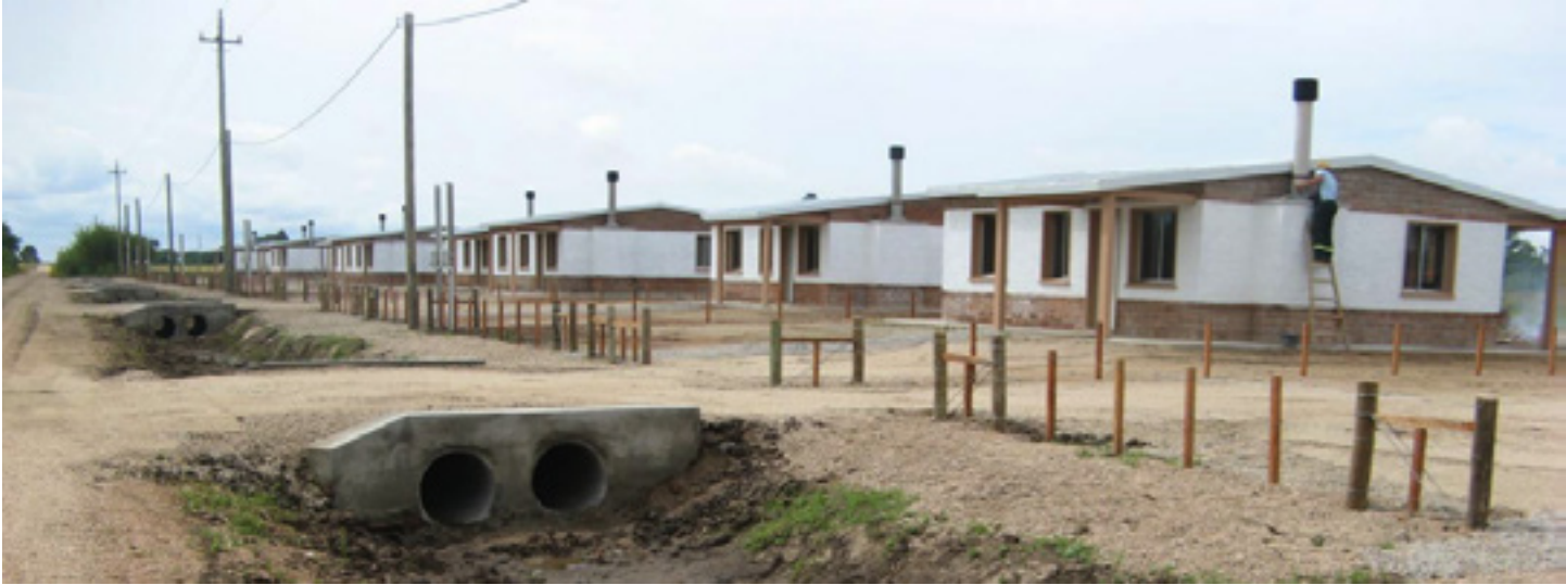
Figure 8: Photo 1st of the new fisherment's housing. Sources: Cabal Claudia. UTE. Email correspondence. September 9, 2015.
