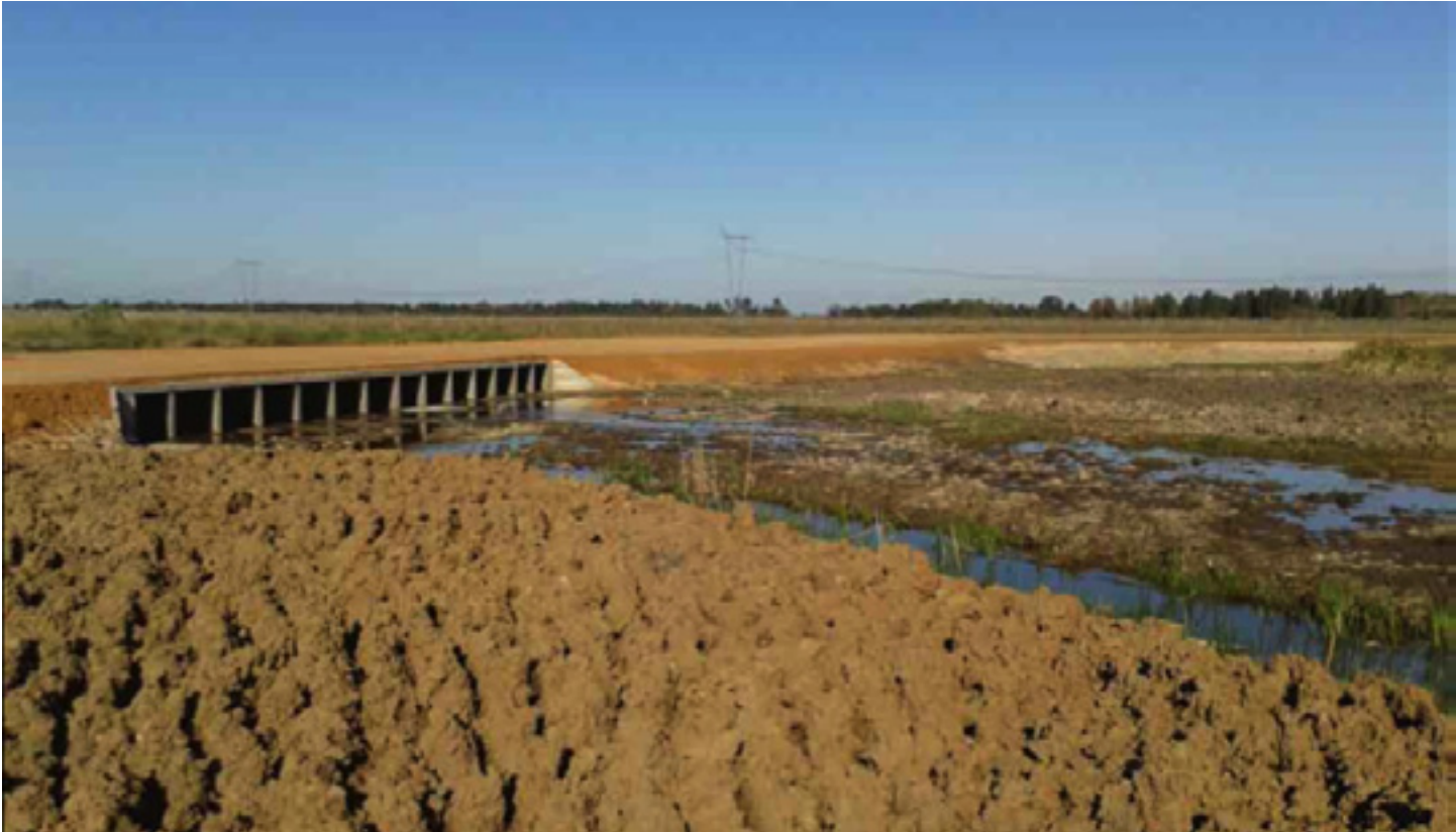
Figure 16: Photo of bridge and road improvements at PTB. Sources: Cabal Claudia. UTE. Email correspondence. September 9, 2015.
