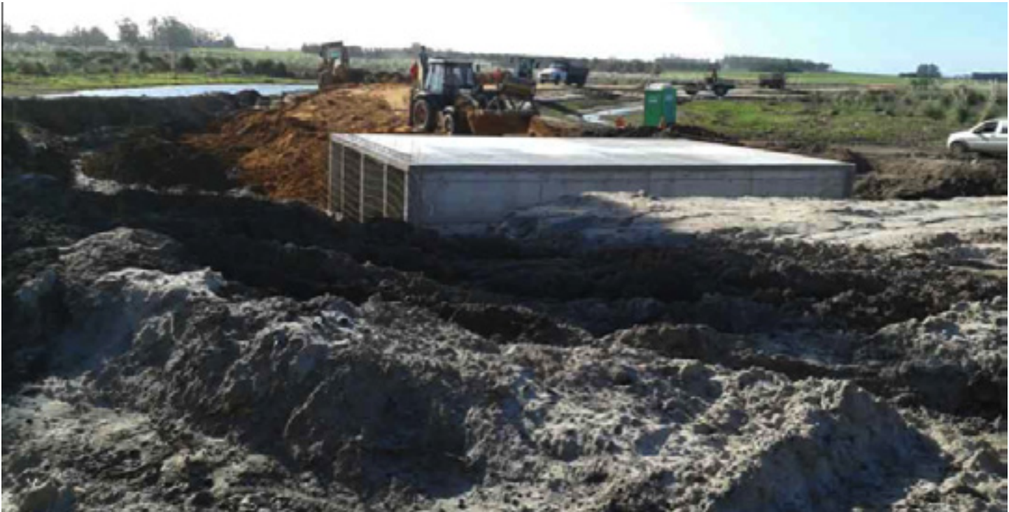
Figure 17: Photo of construction works during road improvement at PTB. Sources: Cabal Claudia. UTE. Email correspondence. September 9, 2015.
