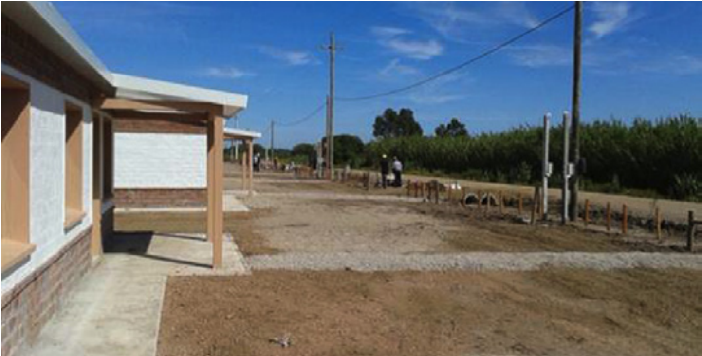
Figure 10: Photo 3d of the new fisherment's housing. Sources: Cabal Claudia. UTE. Email correspondence. September 9, 2015.
