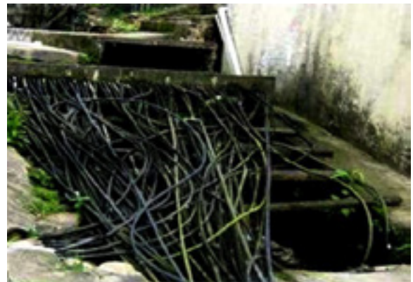
Figure 10: Water supply in a Bairro Cota settlement in Serra do Mar State Park pre-resettlement and urbanization program.
