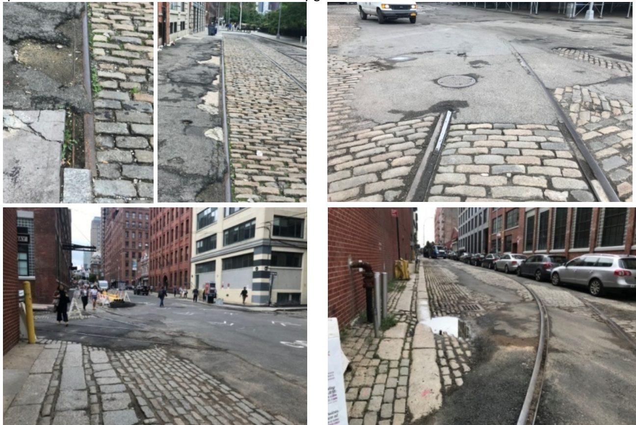
Fig. 3, 4, 5, 6 7: Patchwork-look roadways resulting from piecemeal repaving work done over many years
