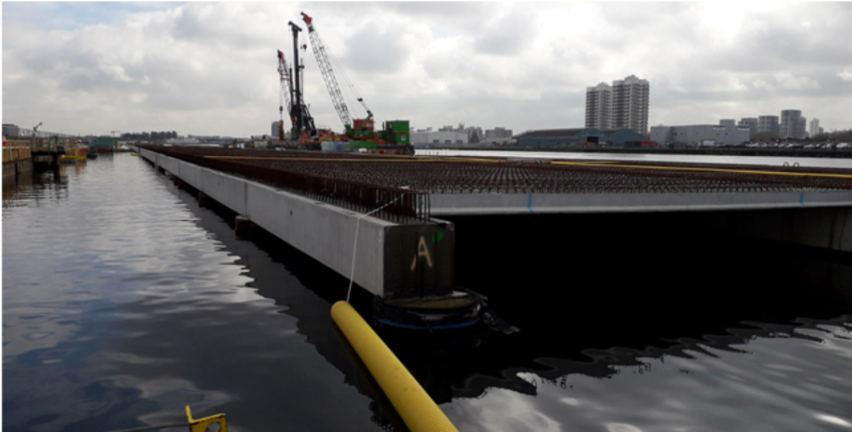
Fig. 26: Piling and deck works over King George V Dock (source: BAM Nuttall)
