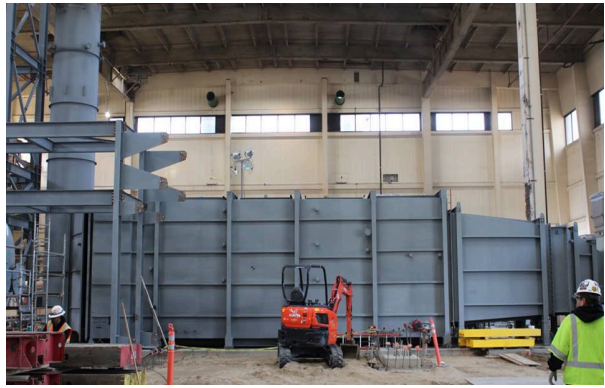
Figure 6: 1 of 2 heat recovery steam generators/Photo from LA Bureau of Sanitation
