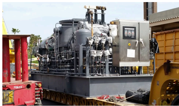
Figure 7: 1 of 2 steam turbine generators/Photo from LA Bureau of Sanitation
