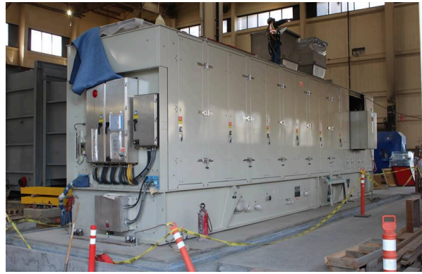
Figure 5: 1 of 2 combustion turbine generators/Photo from LA Bureau of Sanitation
