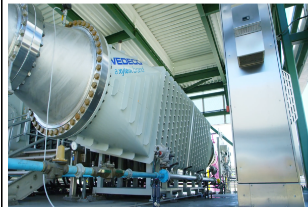
Figure 7: Advanced oxidation process equipment/LA Bureau of Sanitation, 2018
