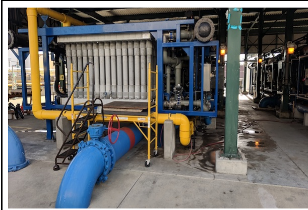
Figure 5: Microfiltration equipment/LA Bureau of Sanitation
